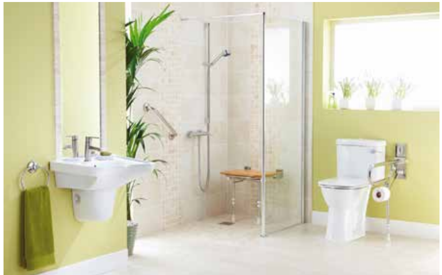
Grab bars and barrier-free showers make the bathroom more accessible. Image provided by authors.
